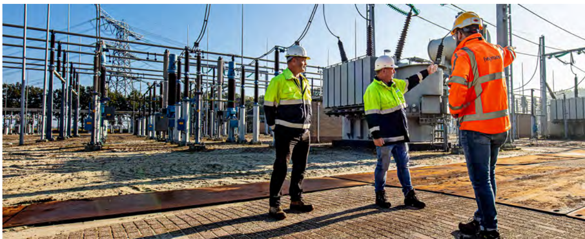
Ingo Seuren of Heijmans with Douwe Zijlstra and construction manager Hans Greven from TenneT at the high-voltage substation in Meeden
